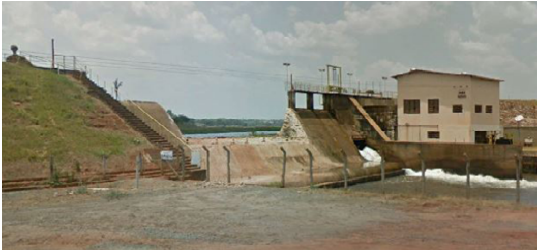
Figure 1 - Front view of the SHP Corujão Dam, in Araguaína - TO (Source: Authors, 2018).
